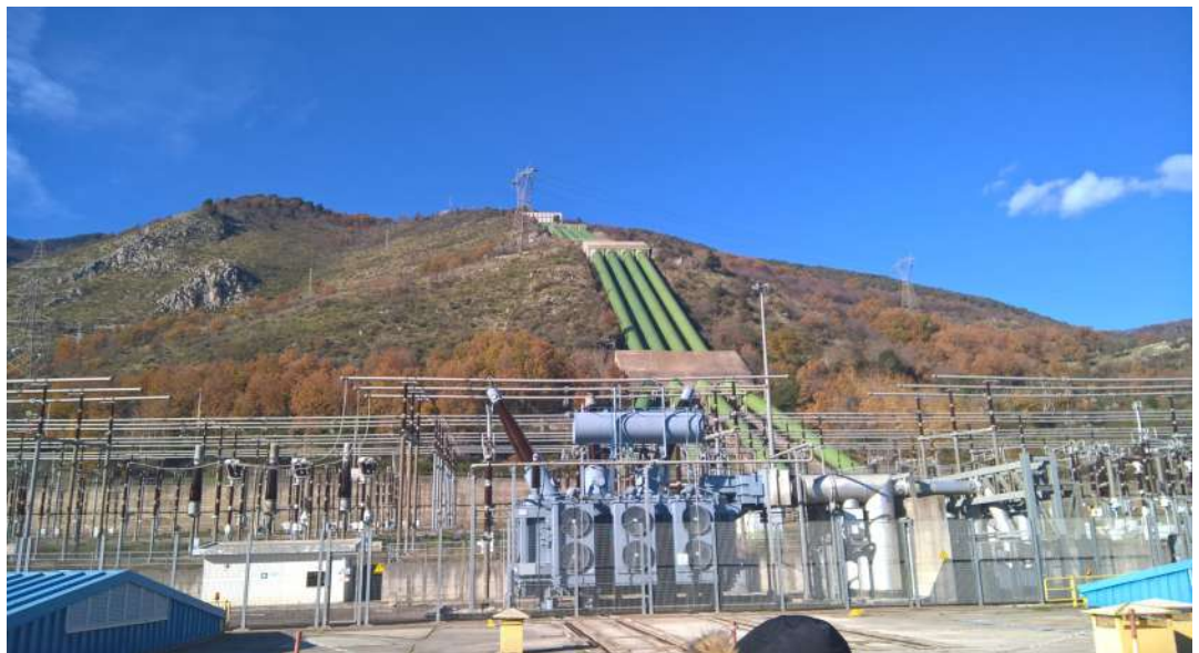
Hydroelectric power plant in Presenzano "Enel" (the National Electric Body)
